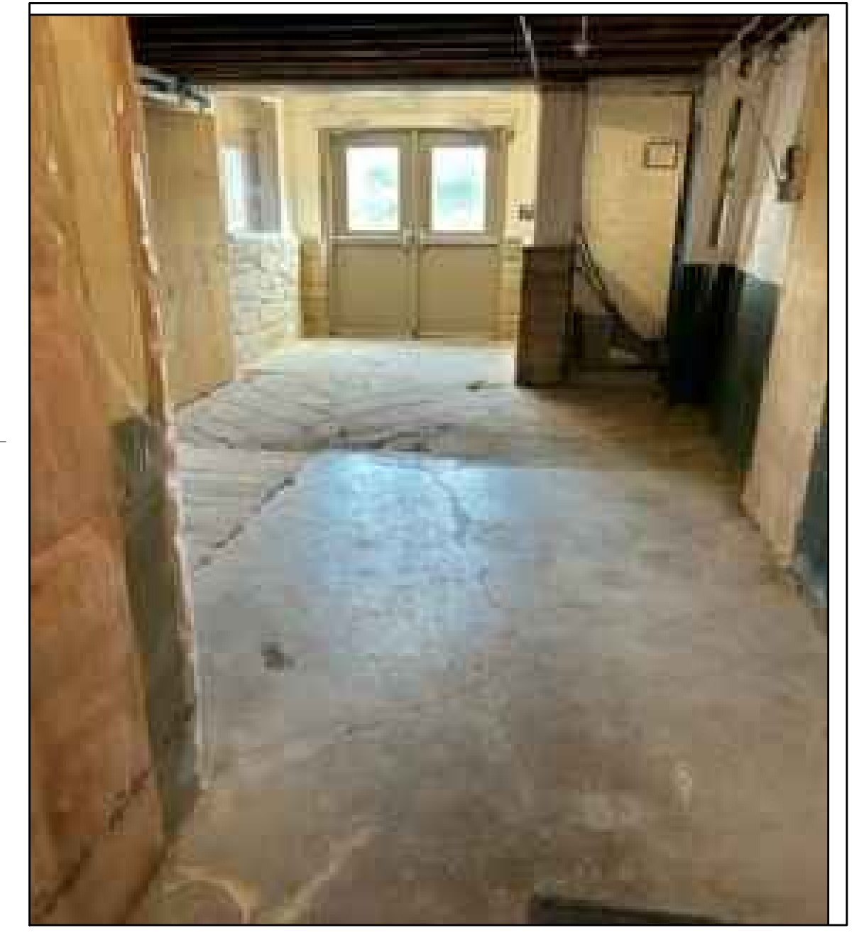
FRONT ENTRANCE FLOOR CONDITION
